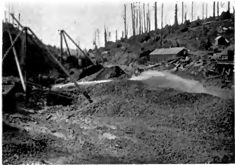
JACOBY CREEK QUARRY — THE LITTLE GIANT MONITOR. PILES OF WASTE ROCK ARE ITS SPORT.
